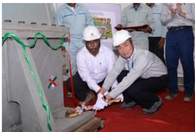
Mr. J.N. Singh, the CEO of MUNPL, and the representative of Toshiba (Power Systems Company) tighten a casing bolt.
