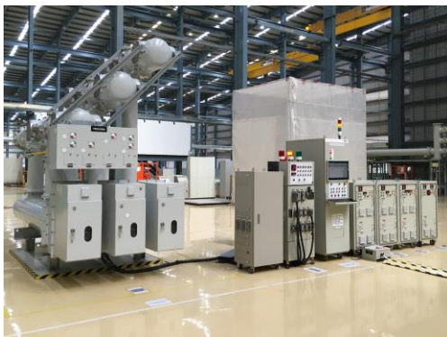
Gas Insulated Switchgear
